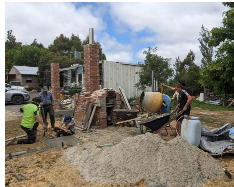
Mountain Track participants Tyson, Geoffry, Alex and Cody helping out a neighbour with a concrete slab pour. Photo Laura Myer
