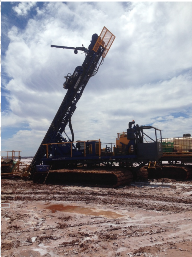
Figure 3 Specialised lake diamond drill rig set up on first hole (looking north)
